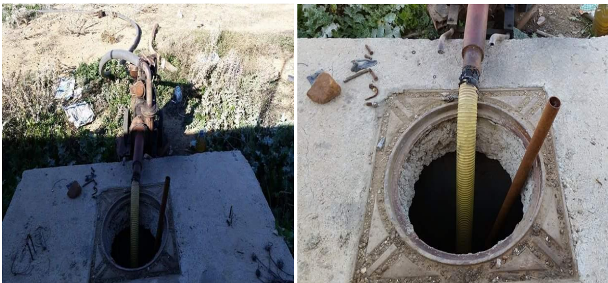
Figure 1. Device for the use of treated wastewater at the outlet of the treatment plant.
